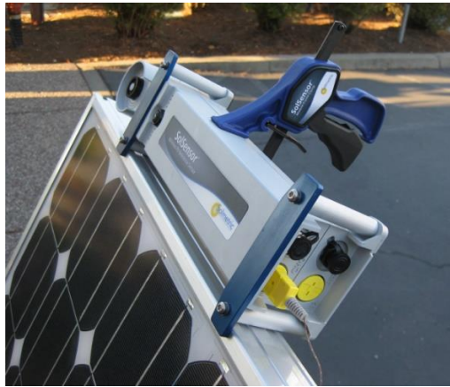
Figure 20. SolSensor mounted on the frame of a PV module
